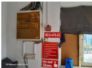
Centralised Fire Control Panel.jpg
