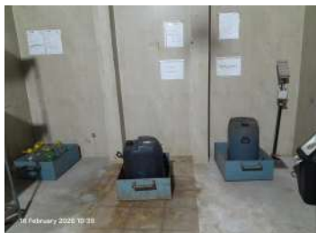
Domestic Chemical Store.jpg
